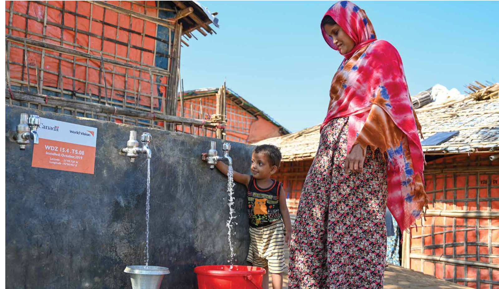
Funded by Global Affairs Canada, this solar-powered network delivers water to 5,000 refugees.
